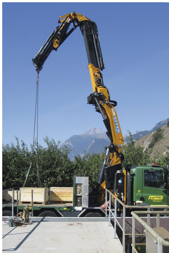
The microbial fuel cell arrives at the Châteauneuf wastewater treatment plant in Sion. Photo: HES-SO Valais
